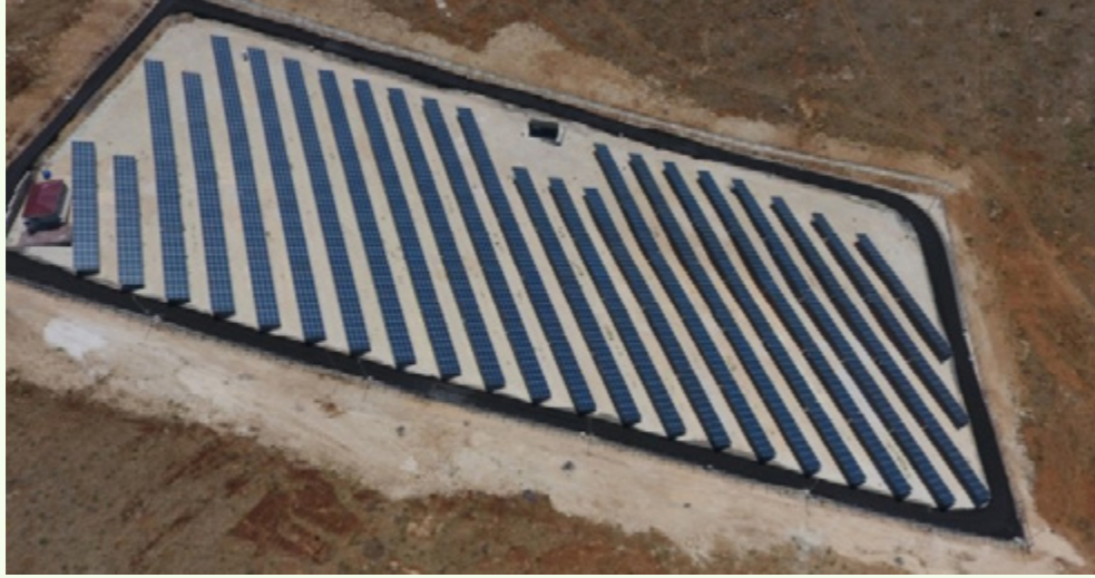
Figure 9. Gaziantep Metropolitan Municipality Bağlarbaşı Solar Energy Power Plant.
