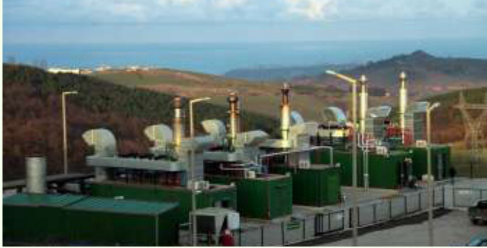
Figure 11. Landfill Gas to Electricity and Sludge fed Cogeneration Plant in Samsun 191
